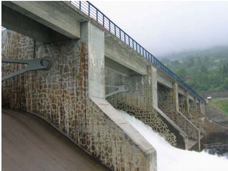
Figure 2.1: ASR affected dam in Norway (Thomas 2013)
